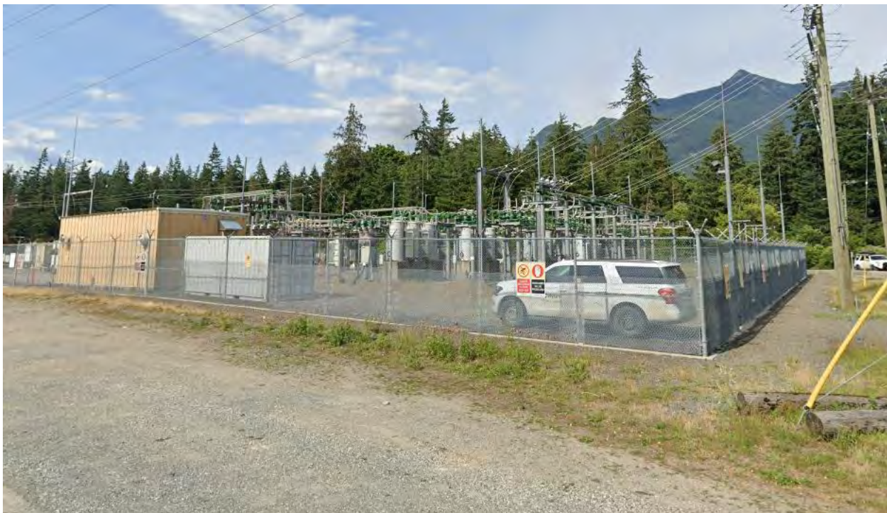
Photo 6. BC Hydro substation on 7 th Ave.
