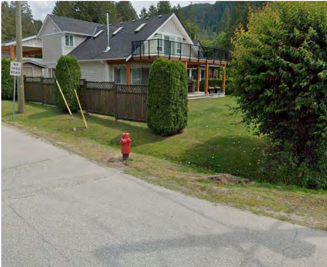
Photo 5. Hydrants in the Kawkawa Zone may not provide sufficient water supply for fire suppression.
